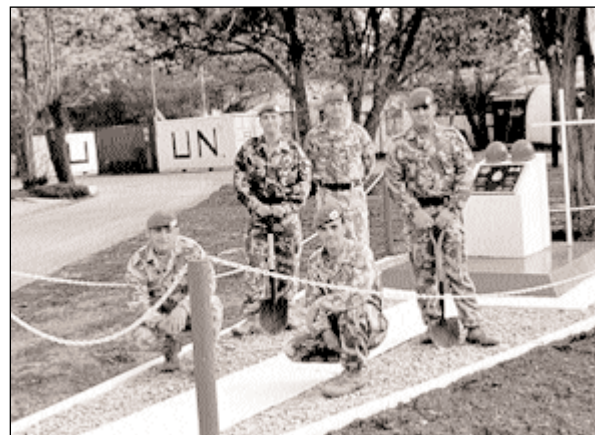
The MT cell at the CANCON memorial, after the renovation was completed
